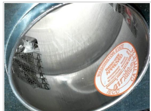
R402.4.4 Recessed Lighting Labeled and sealed recessed light
